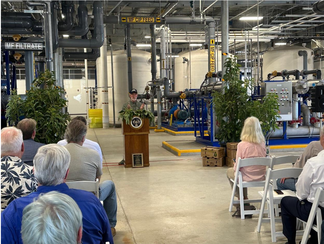
Eddie Grangetto speaks at Escondido’s Membrane Filtration Reverse Osmosis (MFRO) dedication ceremony
